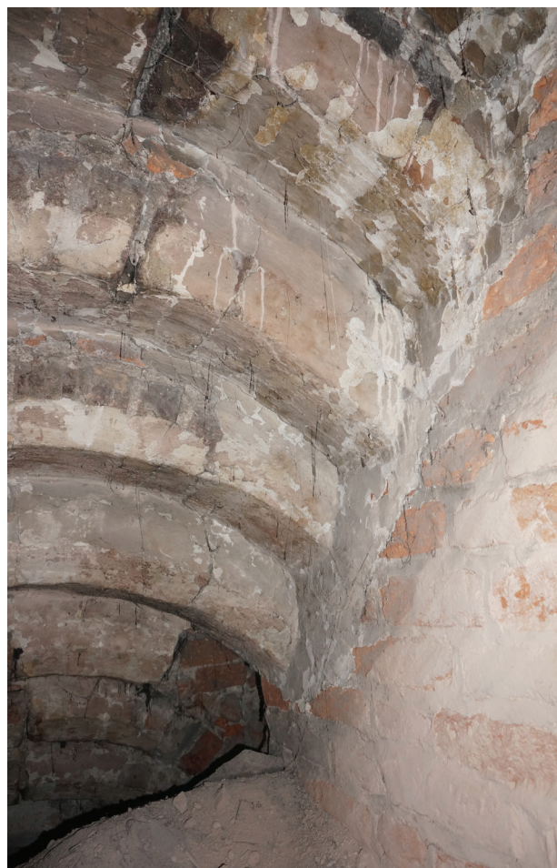
Fig. 5. A section of a partially buried descent from the level of the former matroneum to the ground floor of the chapel at St. Joseph's Church in Gdańsk (photo by A. Piwek)
