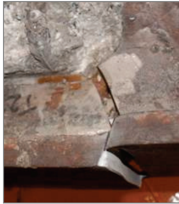
Fig. 6. Considered crack after concrete is partially removed
