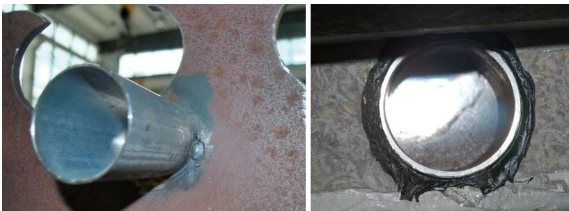
Fig. 38. Channel before concreting and view through the channel after concrete is casted
