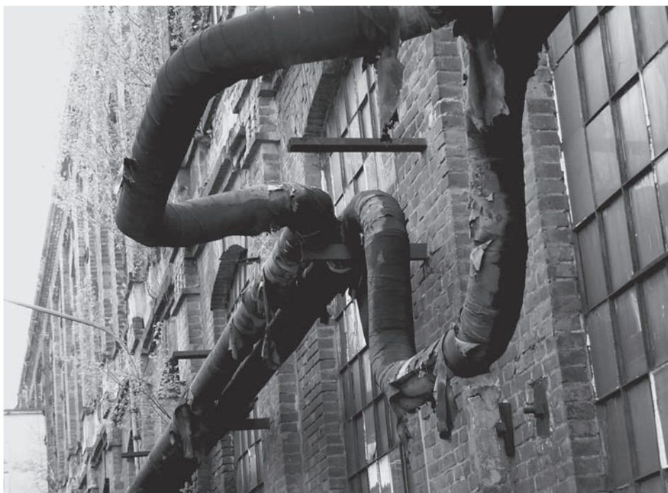
Fig. 5. Façade detail showing the present condition of buildings in Sheibler complex. Photo by M. Rusnak, 2010
