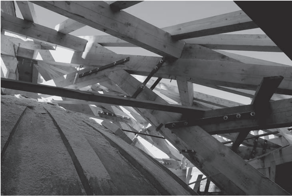
Fig. 4. One of the fixing stages of the roof truss above the presbytery
