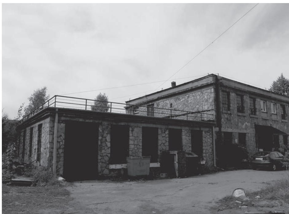
Fig. 10. Skarżysko-Kamienna. The remains of postindustrial buildings of State Factory of Ammunition (PFA) localized in the forest. Its urban layout is specific for residential with street planted with trees and roofs covered by greenery. Photo by author, 2010
