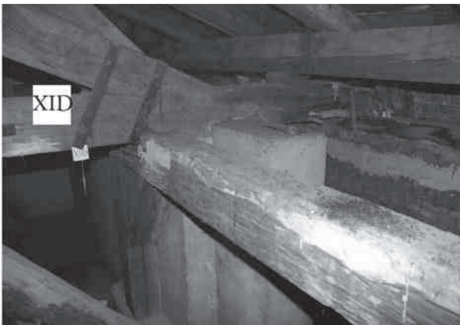
Fig. 4. Markings of various types of main trusses and places of destruction
