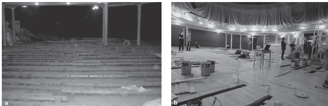
Fig. 3. Replacement of floor construction in 2008: a) floor joists placed on reinforced concrete floor; b) parquet floor boards on plywood and joists
