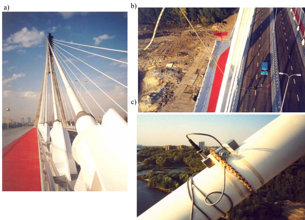
Fig. 12. Cable-stayed bridge over the Vistula River in Warsaw: a) pylon and cable system, b) cable deflection applying c) accelerometers in the middle of cable length
