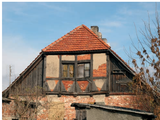
Fig. 2. Granecznik, examples of damage caused by a lack of current repairs and maintenance of wood
