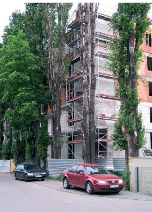
Fig. 4. Drastically topped, preserved despite a collision Populus nigra Italica at arising building ul. Reja in Wrocław (photo by B. Malczewska, 2006)
