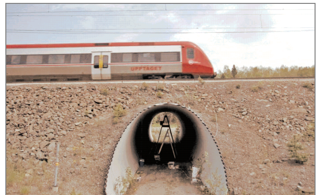
Fig. 1. The passage of a train along a soil-steel structure in a dynamic test [4]
