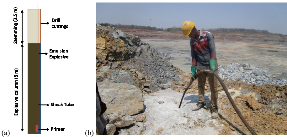
Fig. 2. (a) Vertical section of the blast hole charged with SME, (b) Snapshot of charging process
